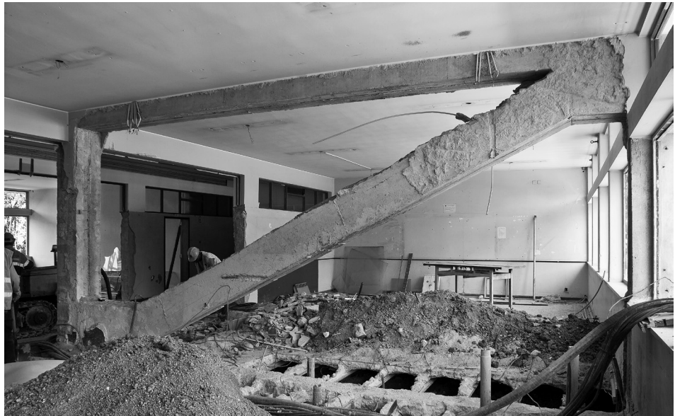
Figure 8: Liceu de Rainha D. Leonor (1957-1961), Lisbon. Diagonal structural element in reinforced concrete portico designed to ensure adequate seismic resistance of the building in the transverse direction.
